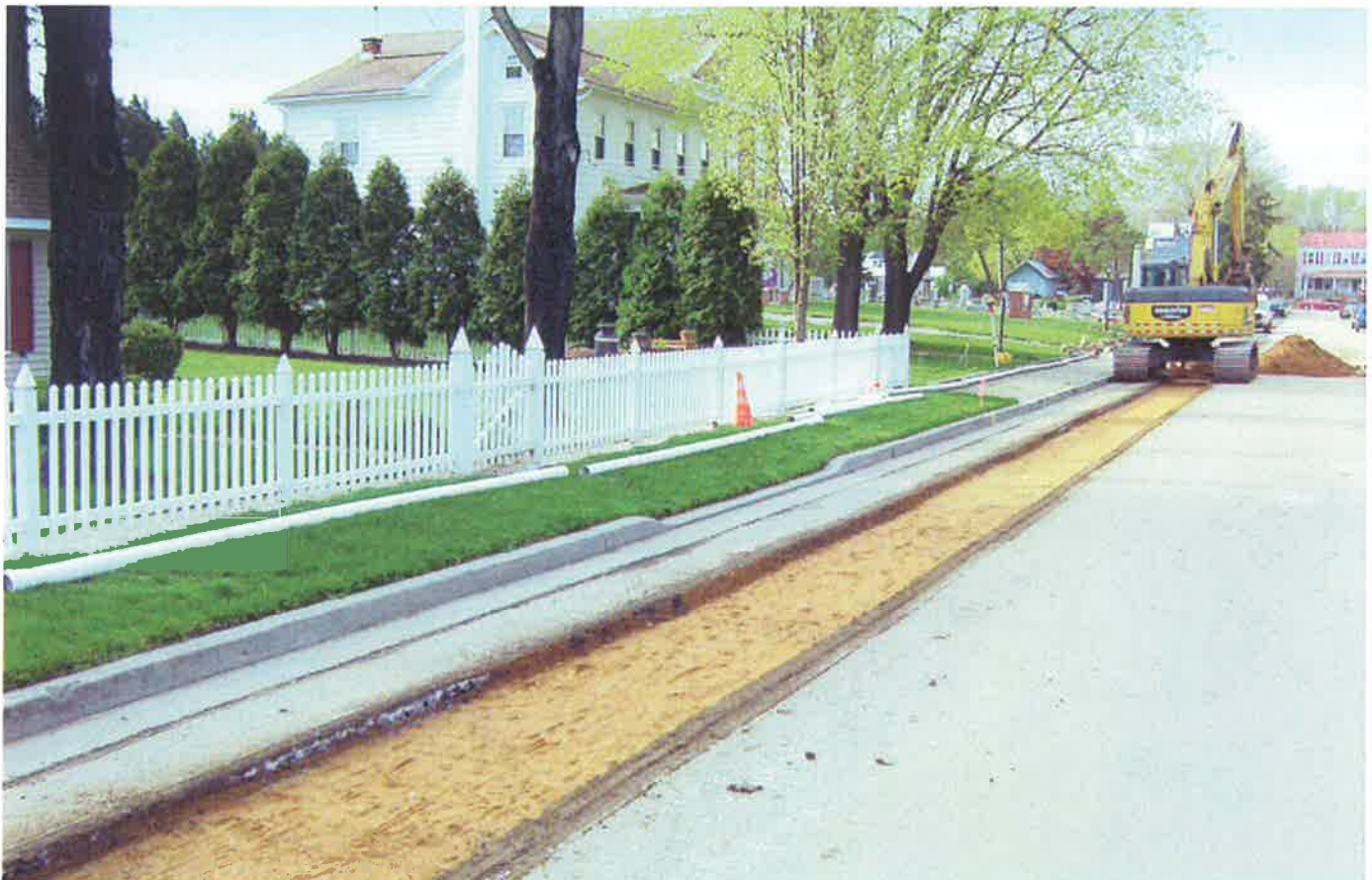
Vacuum sewer installation causes minimal disruption to neighborhoods. Trenches are shallower, less excavation is required and streets can remain open to traffic.
