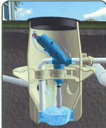
1 Traditional gravity lines carry wastewater from the customer to an AIRVAC valve pit package.
