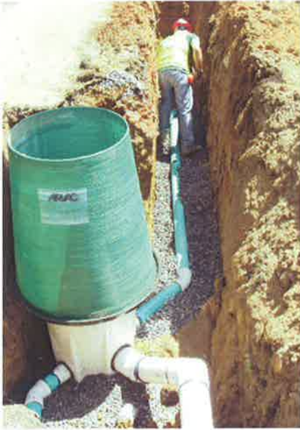
Gravity lines transport sewage from the home just like they do in a gravity system, but at the street or property line, the sewage empties into a buried valve pit.
